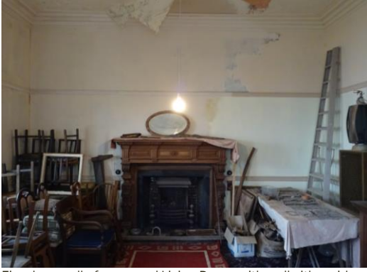
Fireplace wall of proposed Living Room with wall either side of the fireplace for proposed jib doors
