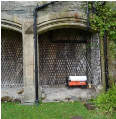
One of the two archways on the south elevation (second to left)
