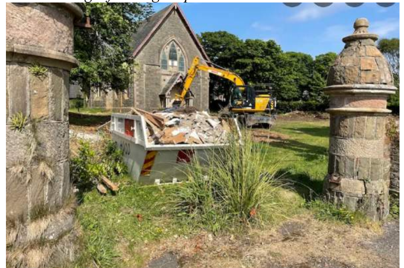
Deteriorating left-side gate-pier 2021
