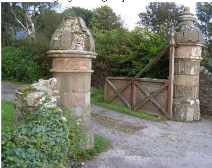
Craigrownie Church Damaged gate piers (10/9/2009) © Scottish Civic Trust
